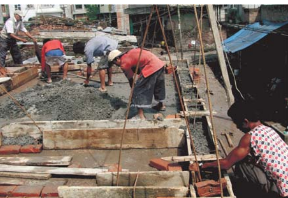
Construction of first floor at Buddha Jyoti Bal Udhyan LSS, Balaju, Kathmandu under SESP/DRRSP/Action Aid Nepal
