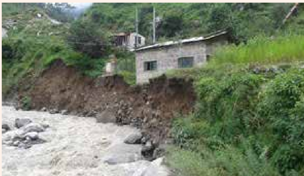
Figure 4 Power house of the Triveni Micro Hydropower Project at risk by the Bahuli Rivulet, in Martadi of Bajura (Source: Prakash Singh) http://www.the-himalayantimes.com/fullNews.php?headline=Bajura+headquarters+in+dark+for+five+days&NewsID=424456#sthash.77OQPrqW.dpuf
