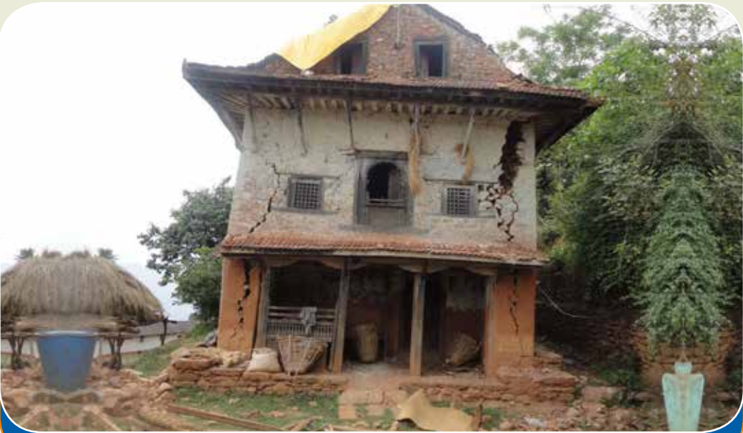
A Rural House Damaged by Gorkha Earthquake
