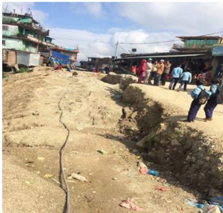
Pic 2: Highway that runs through Kapurkot Municipality has a major creeping landslide. Seen here in a differential settlement along the highway. The cracks along the road are reported to be increasing every year. Pic: Survey Team.
