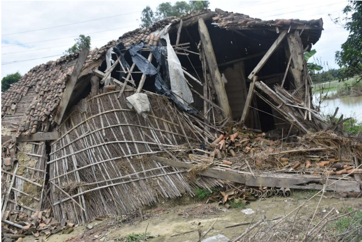
Damaged house in Samsi Rural Municipality. Photo by Bhesh Parajuli on July 28, 2019.
