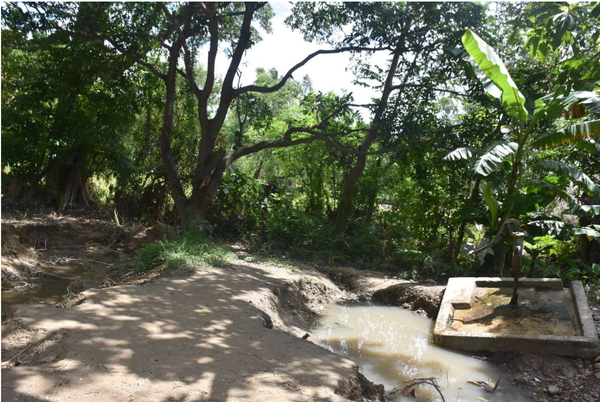
Damages on tube well in Samsi Rural Municipality. Photo by Bhesh Parajuli on July 28, 2019.
