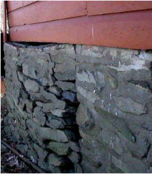
F.3 Bulged and leaning stone Foundation
