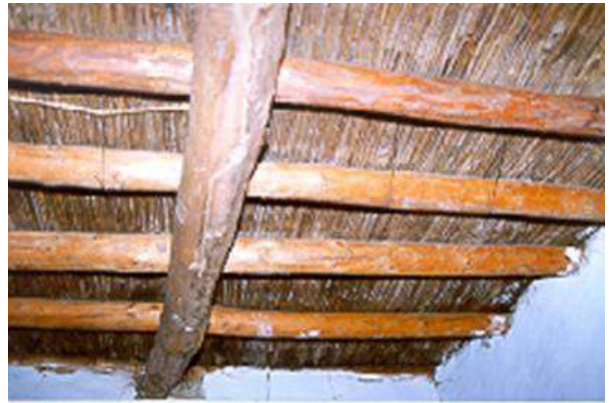
R.4.2 Inadequate and poor floor members
