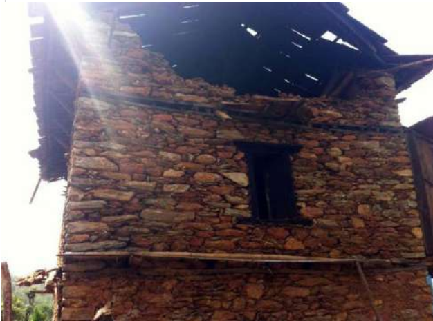
R1.1 Gable wall toppling
