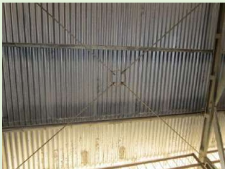
Diagonal Steel bracing to roof
