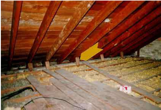
R.4.1 view inside the attic showing the rafters and the absence of collar beams and joist connections to the rafters
