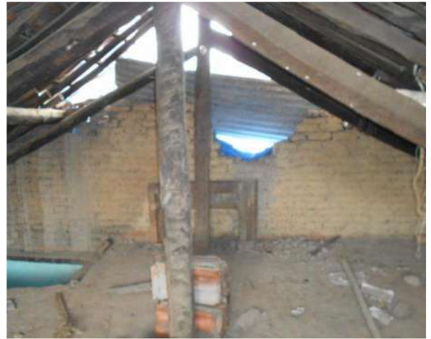
R.1.2 Gable wall toppling
